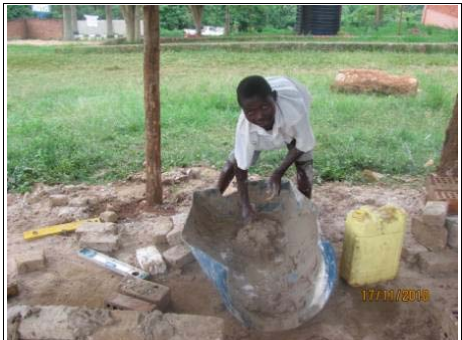
Dan Ssekisambu mixing sand and cement to starting the building lesson at RYDA centre
